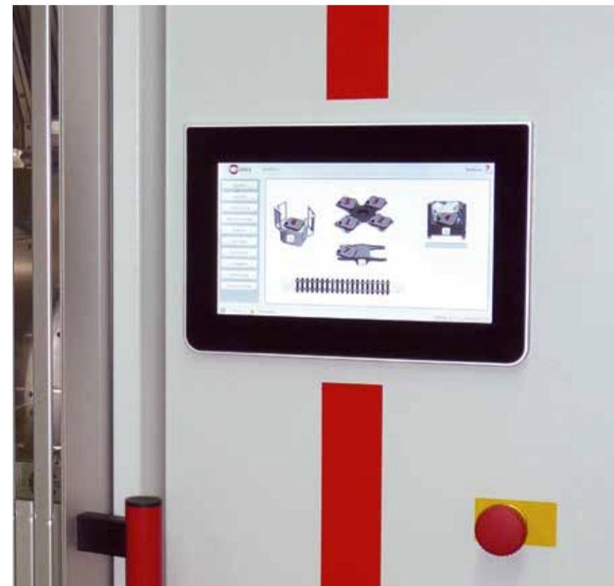
The additional control panel - adapted to the pallet changer setup station.
